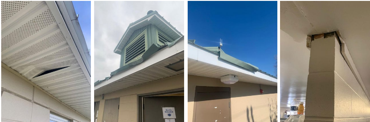
Figure 2. Images of structural damages sustained at facilities that housed Afghan Refugees at Camp Atterbury, Indiana Source: The Indiana National Guard.
